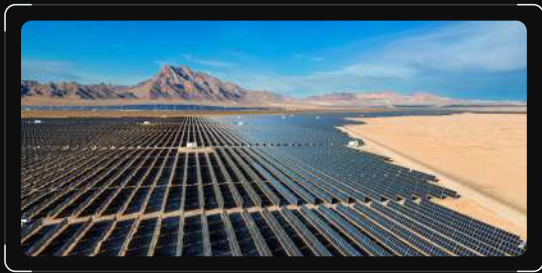
— ARRAY OF SOLAR PANELS IN NEVADAN DESERT
