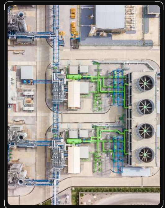
-- AERIAL VIEW OF ELECTRIC SUBSTATION
