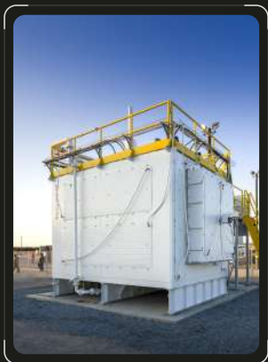
— ANTORA'S THERMAL ENERGY STORAGE SITE IN FRESNO, CALIFORNIA
