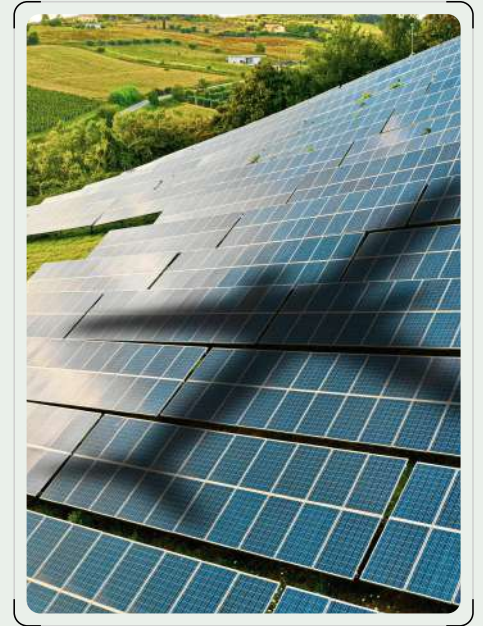
THE SHADOW OF A PLANE AGAINST AN ARRAY OF SOLAR PANELS
